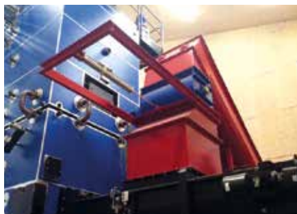
Straw burner feeding system and knife gate for back fire protection.
